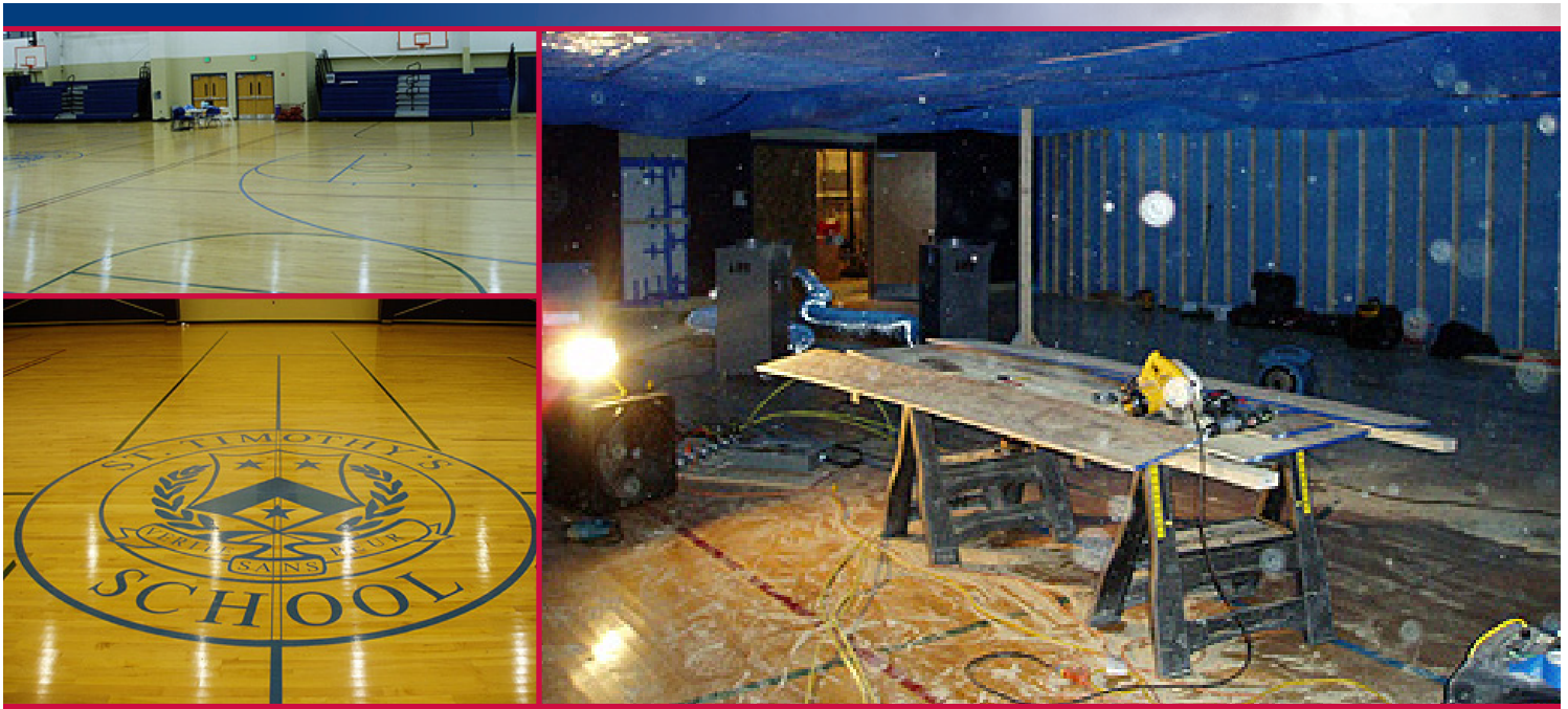
Left Photo (Top): Upon completion of the restoration project, the entire gym floor was sanded and re-finished.
